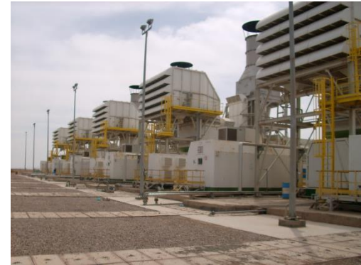
GAS TURBINE POWER PLANTS
