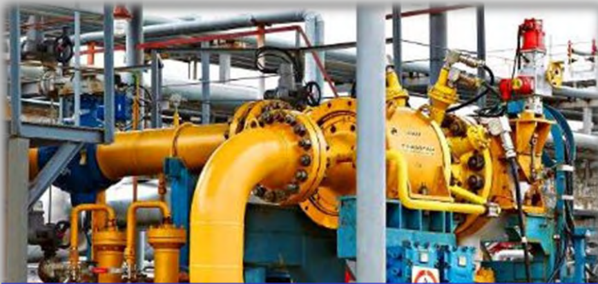
Expander-compressor units for Natural Gas (NG) and associated oil-gas (AG) treatment and processing
