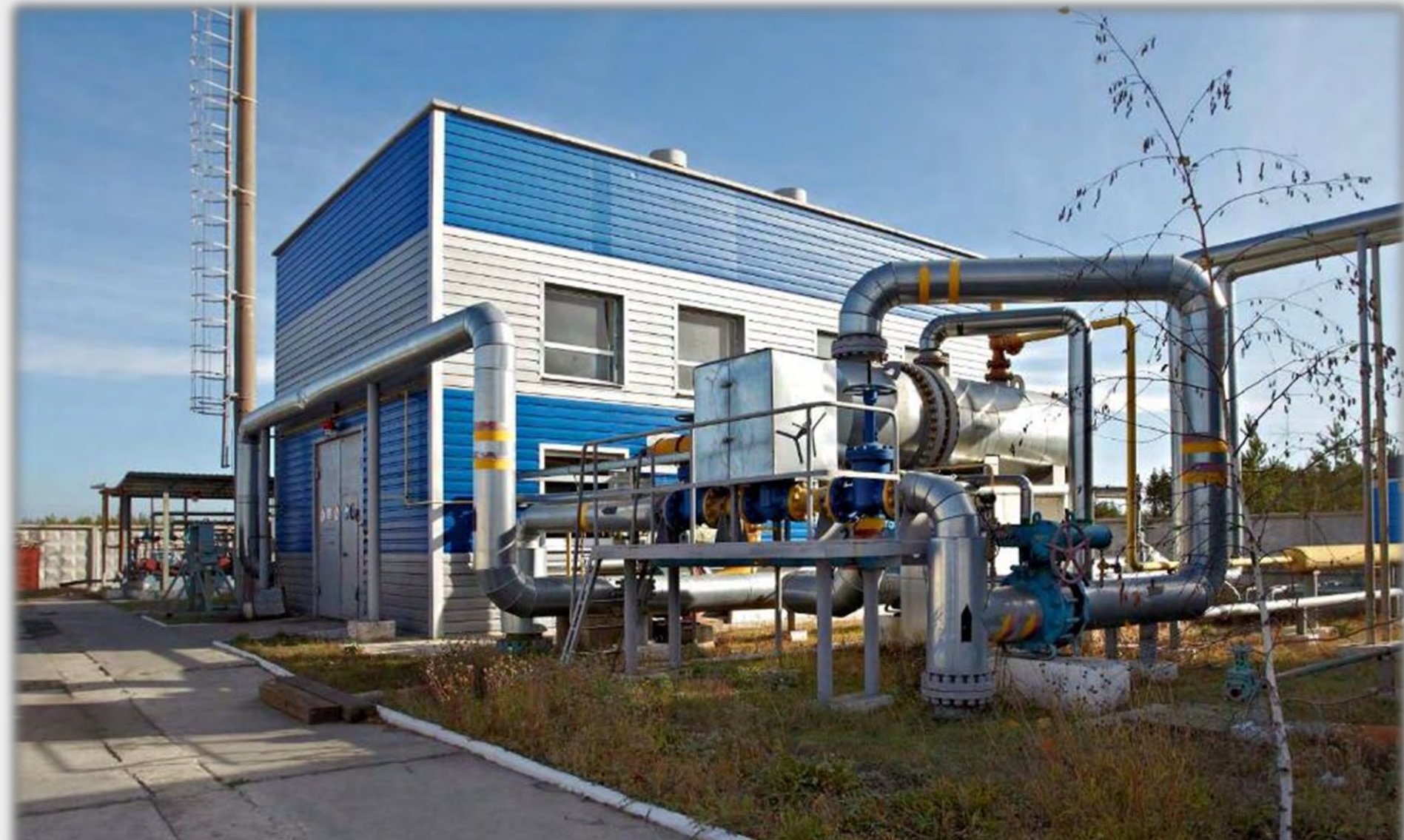
Turboexpander-generator UTDU-4000, 4 MW capacity, UTDU– 4000-4,5-4,5-UHL4 at Severodonetsk gas distribution station, Ukraine, 2008.
